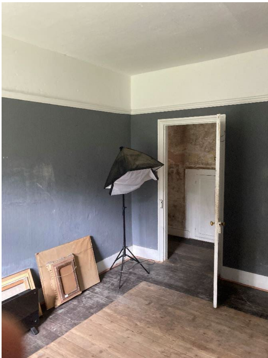
Plate 21: Room 1, new door proposed to be created and doorway blocked but left in-situ
