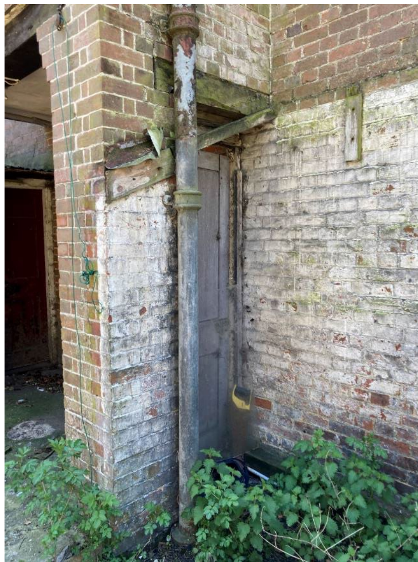
Plate 14: Close up of brick pillar for extension to the rear of the western elevation
